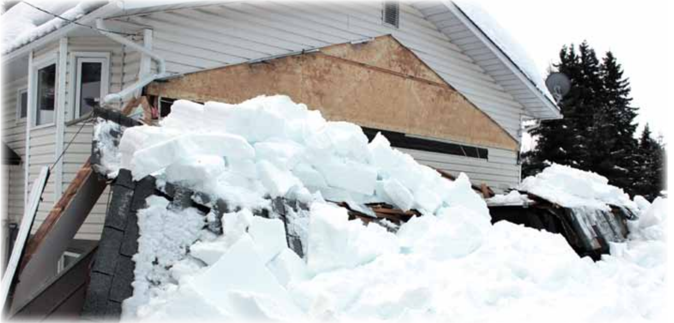
Heavy snowfall this year has caused a series of roof collapses in Idaho.
