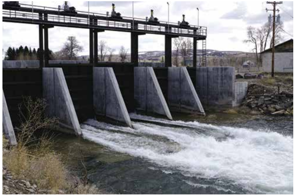
Photo courtesy of Idaho Department of Water Resources A head gate on the Great Feeder Canal releases recharge water during the 2017 recharge season. Idaho recently received a report evaluating options for adding new Upper Snake River Valley recharge capacity.
