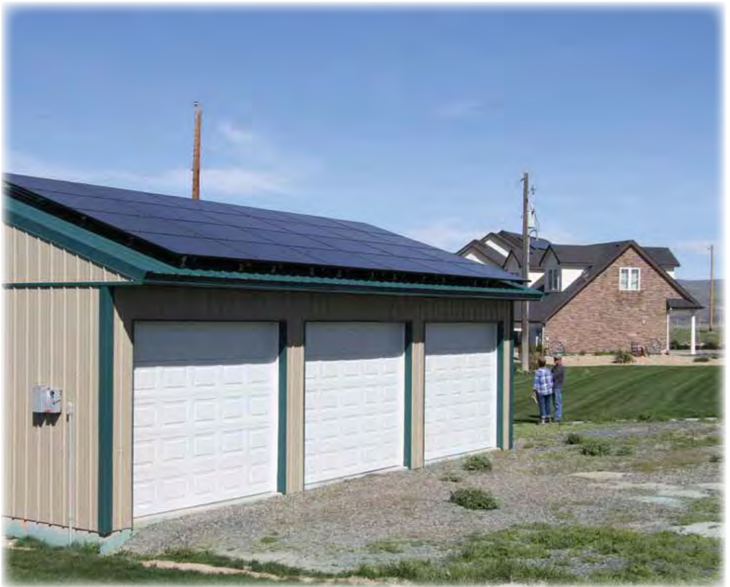
Solar panels installed on the roof of a garage at farm near Melba. Photo by Steve Ritter
