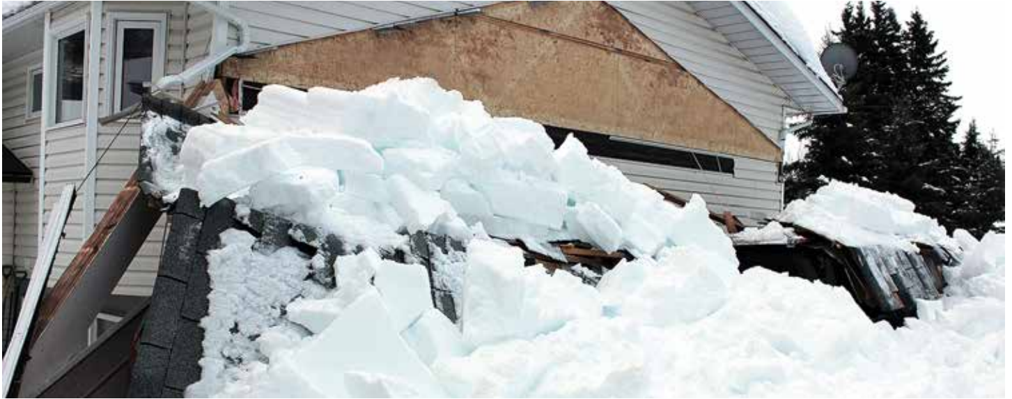
Heavy snowfall in recent years caused a series of roof collapses in Idaho.
