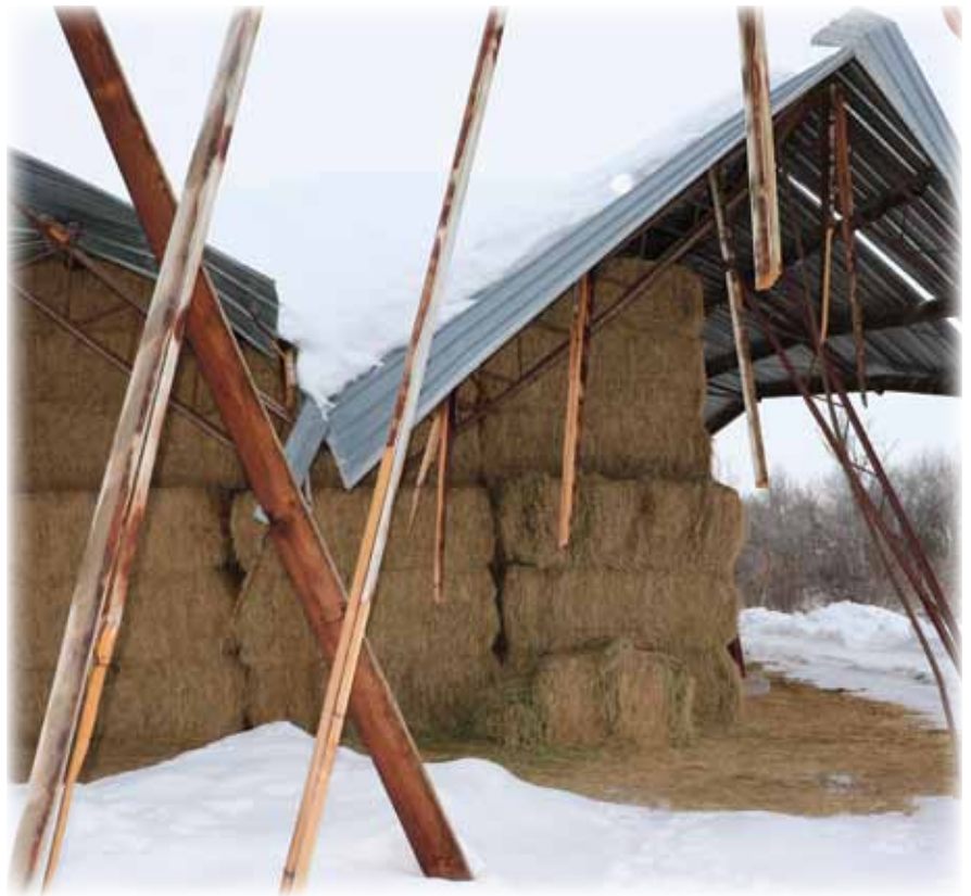
Dozens of hay sheds and other outbuildings were also lost during early January storms.
