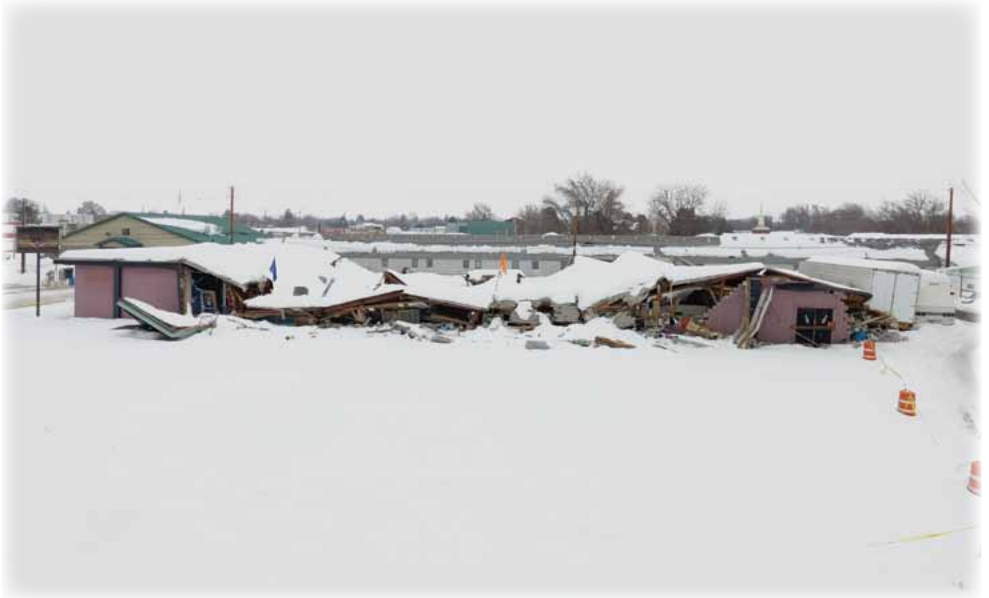
A flattened building in Washington County. Insurance claims adjusters recently confirmed the winter storms that pummeled southwest Idaho in early January resulted in the biggest single event loss in the history of Farm Bureau Mutual Insurance Company of Idaho. Photo by Steve Ritter
