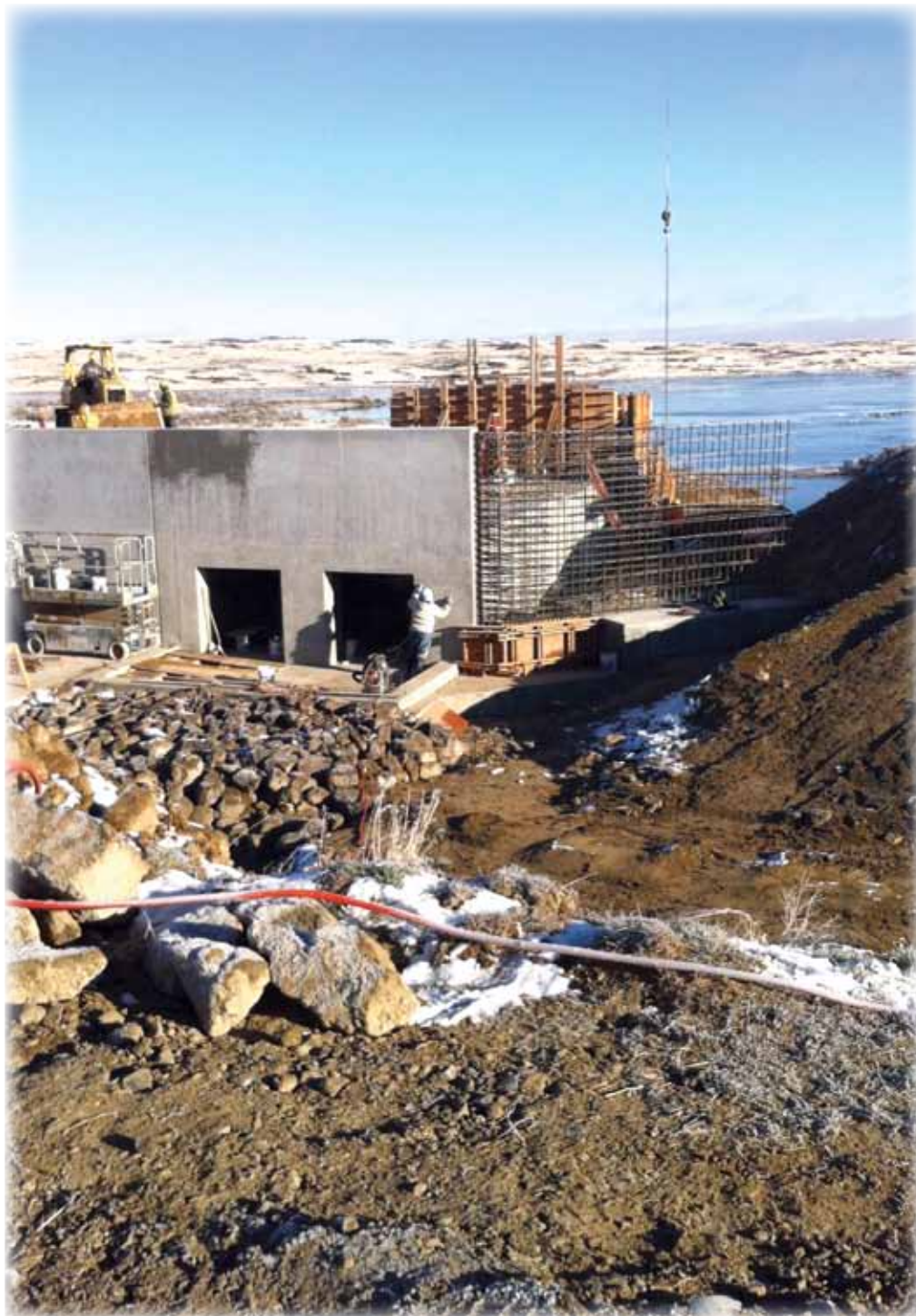
Construction of the new headgates and check dam at the Mile Post 31 Recharge Site last November. Water in the background is recharge that occurred while construction was going on.
